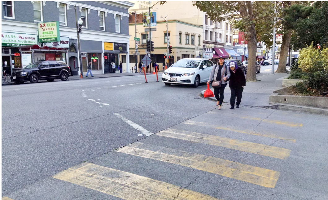
Figure 22. Crosswalk Markings do not Extend to the Curb Ramp Flares
