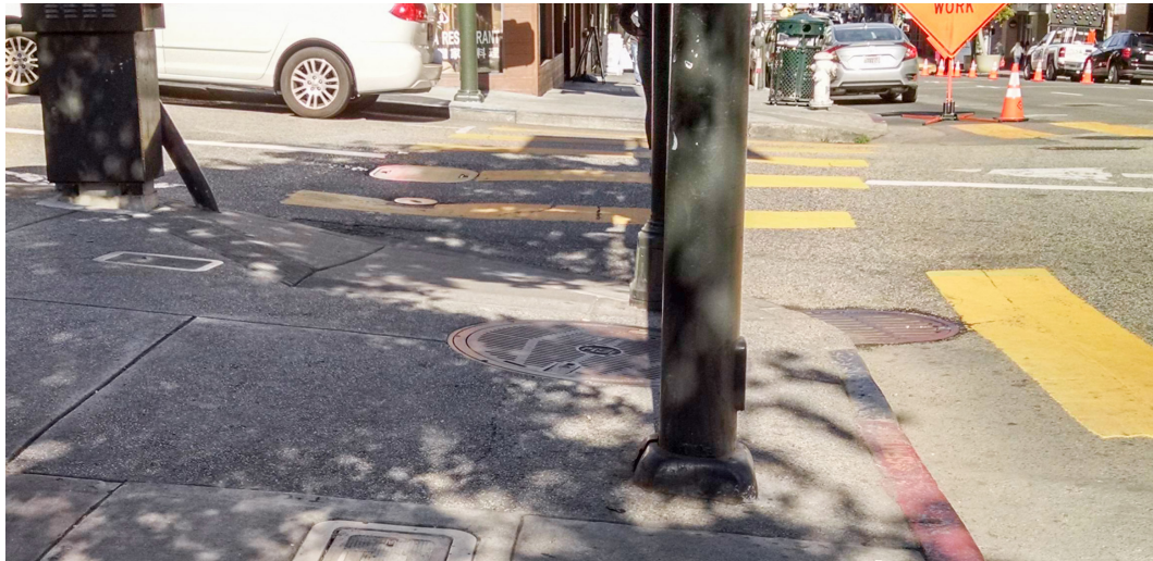
Figure 16. Missing Curb Ramps at Washington Street Due to Utility Conflicts
